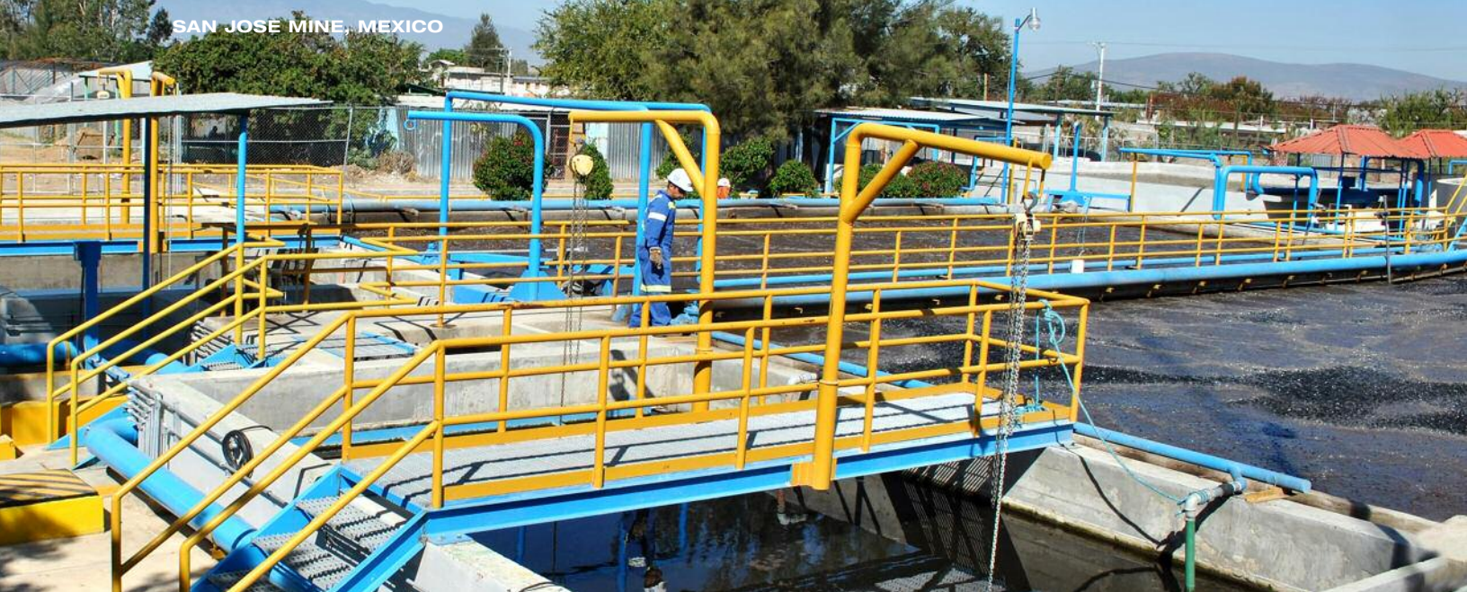
Ocotlan Grey Water Treatment Plant – source of 20% of San Jose's water balance
