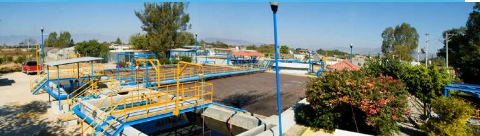
Photo: San Jose Mine- Ocotlan grey water treatment plant
