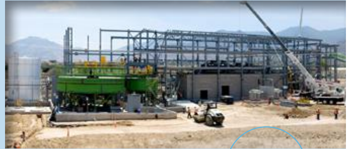
1,500 TPD PROCESSING PLANT
